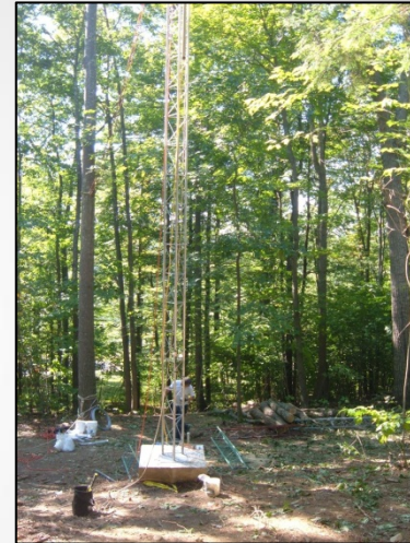
Typical height for a Mast Tower
